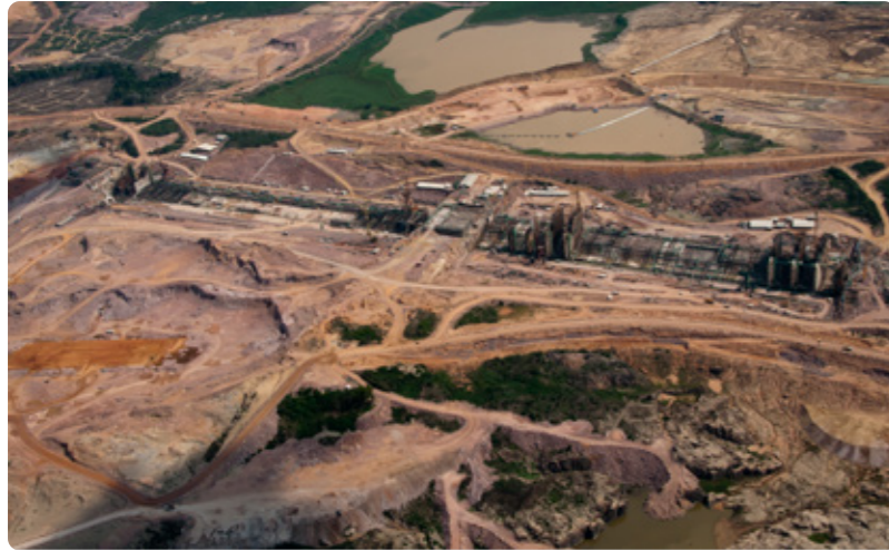
In the last week of January 2011, the mechanical assembly of the spillway began. The first piece installed weighed 30 tons. Four synchronized cranes were used to lift it and fit the 180 metal panels that would form the gates of the water-flow structure. Each unit took, on average, 60 days to be completed
