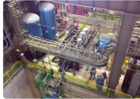
Brazilian and Chinese technicians participate in the test of the armored substation (above and on the opposite page).
