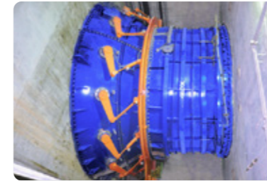
Diagram and real view of Jirau’s bulb turbines. Unlike conventional vertical turbines, this model allows water to flow almost in a straight line through the intake circuit, optimizing energy capture in run-of-river reservoirs with low hydraulic head.
