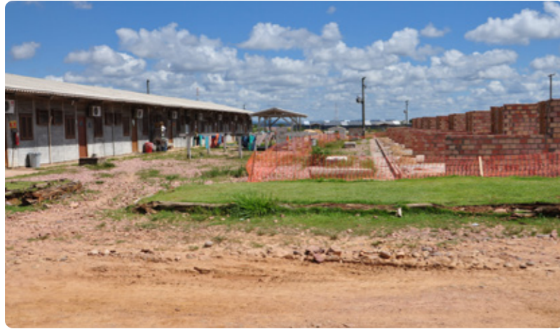
The resumption of the work led to the adoption of temporary modules and mobile kitchens.
