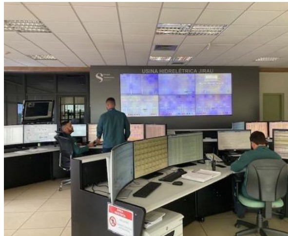
Photo 47: Control room right bank powerhouse
