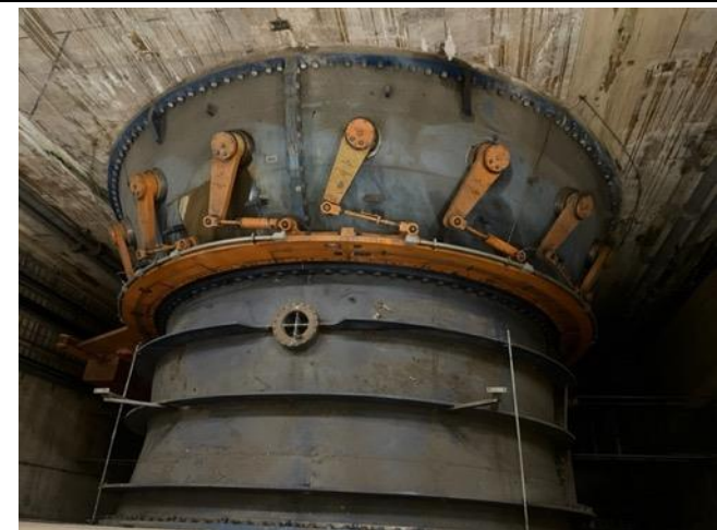
Photo 66: Bulb turbine distributor, view from above
