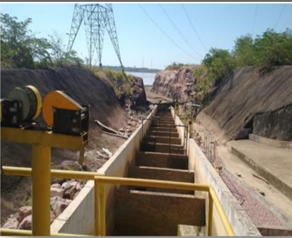
Photo 36: Approach channel of one of two fish passage facilities
