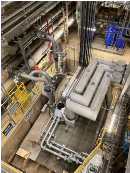
Photo 49: Electrical connections above generator level
