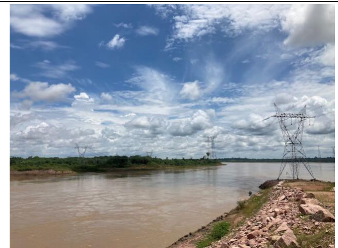
Photo 93: Transmission lines from left bank powerhouse
