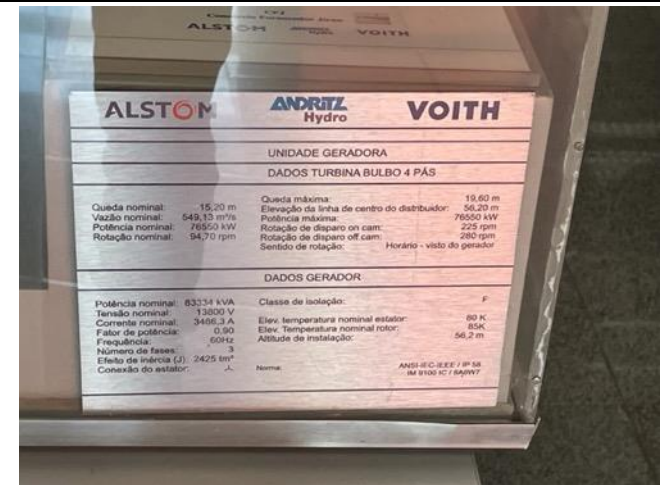
Photo 60: Turbine data right bank powerhouse
